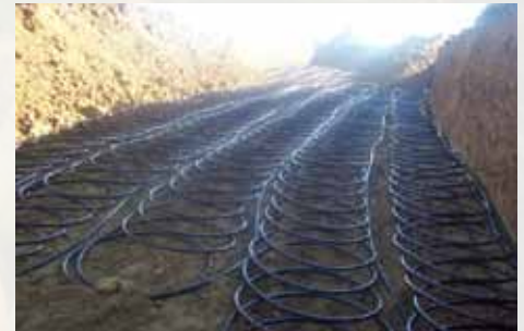
Five out of 20 earth loops used for the Geothermal Greenhouse.
