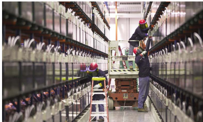
Golden Valley Electric Association, based in Fairbanks, Alaska, uses the world’s most powerful nickel-cadmium battery to hedge against power outages. When needed, the 13,760-battery cell system can provide 27 megawatts of power for 15 minutes.
